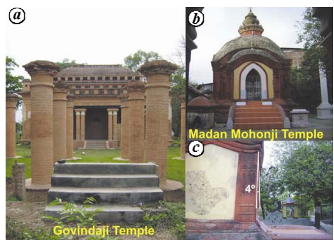
Figure 4. (a) Historical Govindaji temple and the accompanying structure, the Beithoub, in the Kangla palace, Imphal was damaged during the 1869 Cachar earthquake. Other historical temples in the region did not appear to have suffered any damage from the earthquakes. However a small tilt ( \sim 4^\circ ) was observed at the Madan Mohonji temple (b and c) which may not necessarily be ascribed to the earthquake.
